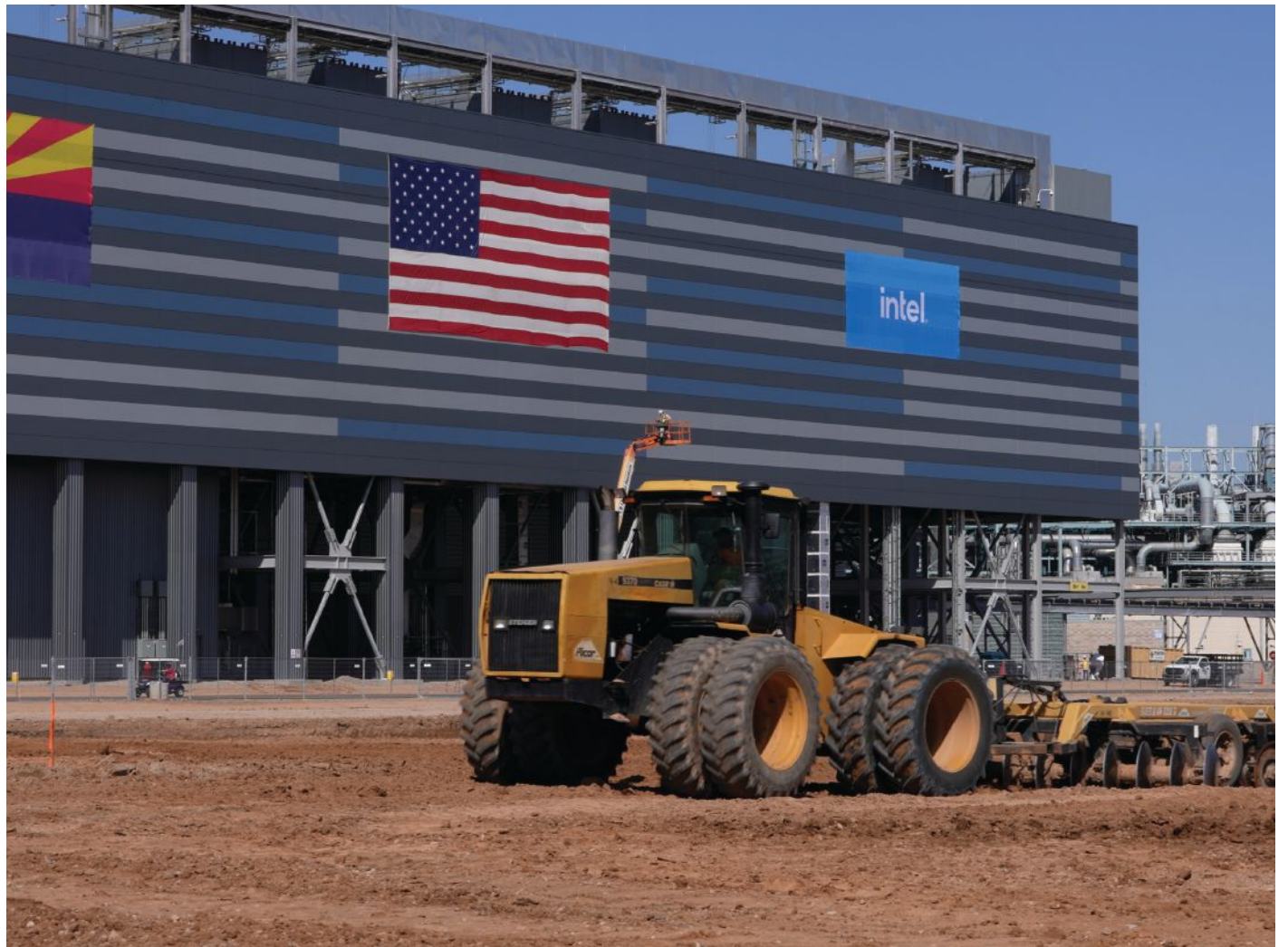
One of Intel's factories at its Ocotillo campus in Chandler, Ariz.
